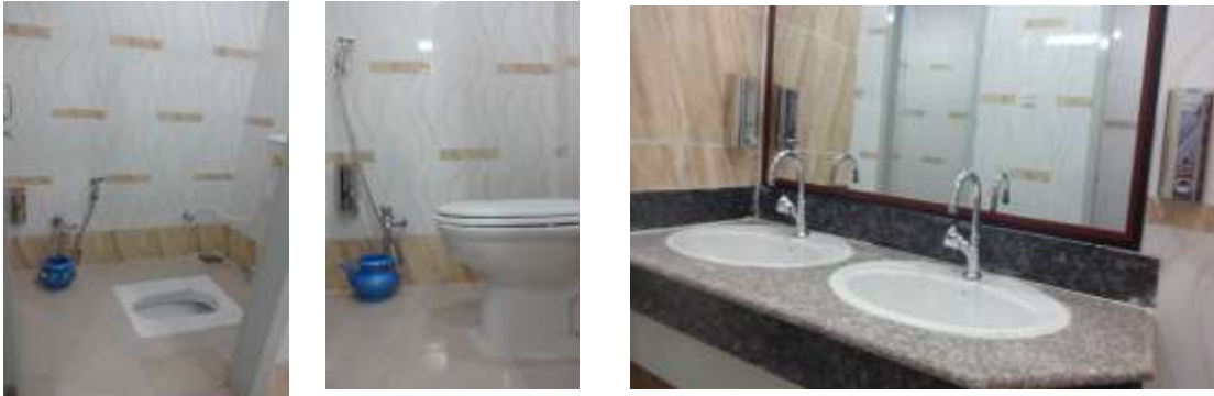
Present normal chamber, High Commode chamber and Hand washing station
