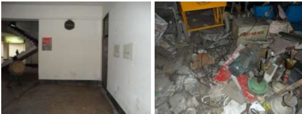
Entrance and the condition of the waiting room inside the bus terminal
