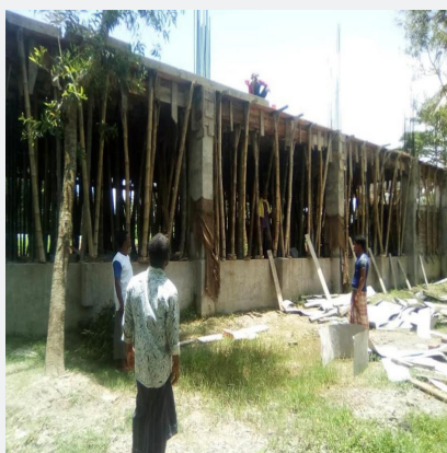
Supervision of work by members of citizen monitoring committee in Keshabpur, Jashore.
