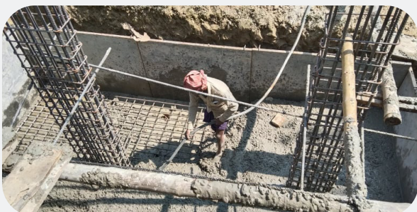
Inspection of base casting of Saldair Khidrogoprekhi Government Primary school in Belkuchi of Sirajganj.
